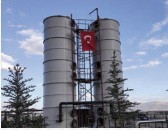
AFYON ARMATECH ENERJİ BİYOGAZ SANTRALİ ARMATEC ENERJİ AFYON
